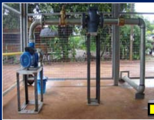
Water pump and valve system
